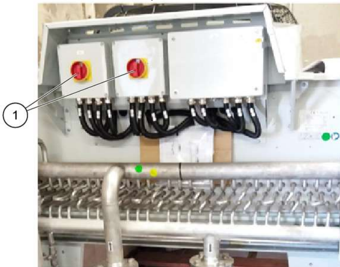
1. Safety switches to fan motors
